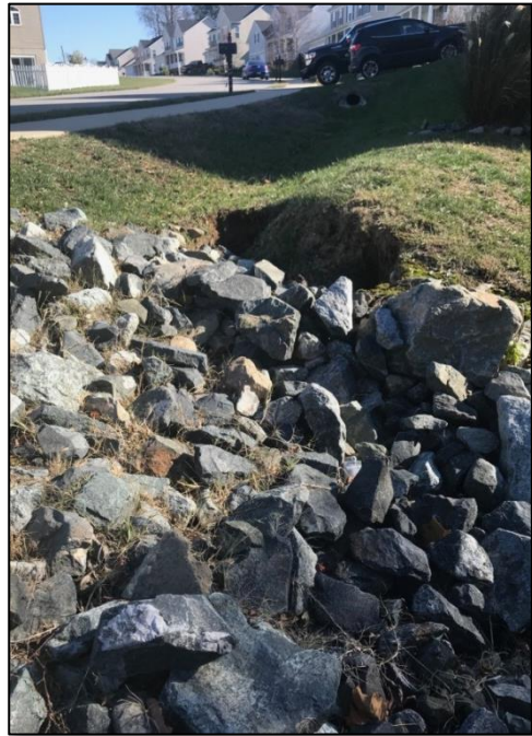
A sinkhole continues to grow near 3122 Lawrin Court.
